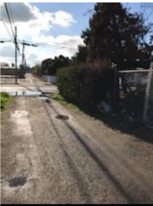
Portion of the alleyway where vegetation would be required to be removed and where the alley would need to be repaved.
